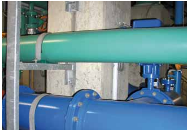
Pipe supports on vertical HZA Channels
